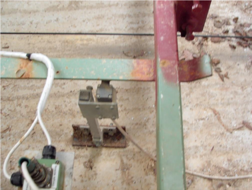
F. Ensure that the skid on the trolley is resting on the limit switch
