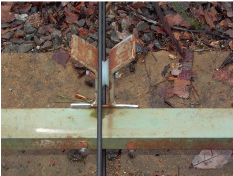
C. Walk down the track and ensure that the drive cable is in the 'Y' pieces and not outside.
