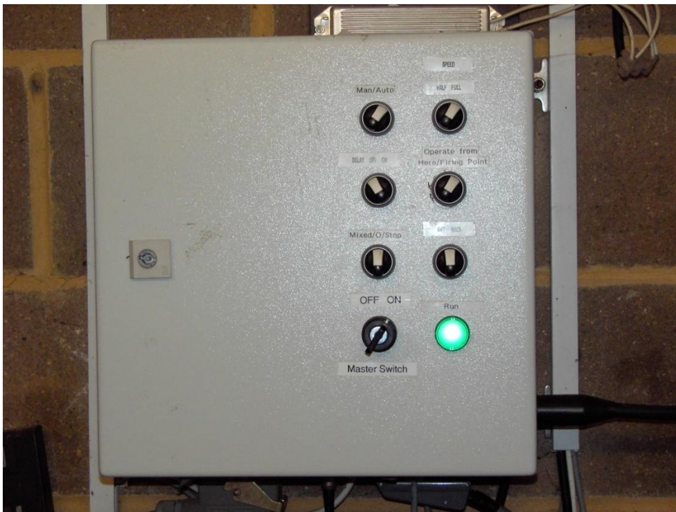
G. This is how the switches should look for normal operation.
